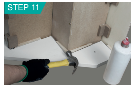
Apply PVA glue to housings in string and knock in wedges tight.
