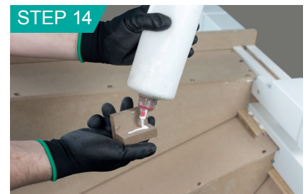
For soffit detail glue blocks need to be fitted to outer joint between tread and riser.
