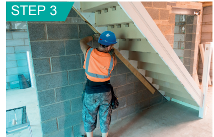
Ensure a packer is fixed to the outer strings to create a gap against the structural wall for plaster finishes.
