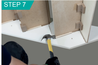
Apply PVA glue to housings in string and knock in wedges tight.
