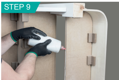
Glue back of tread and routed housing in tread above with PVA.
